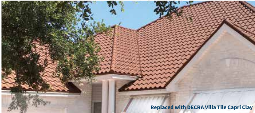
Clay tiles struck by hail.
